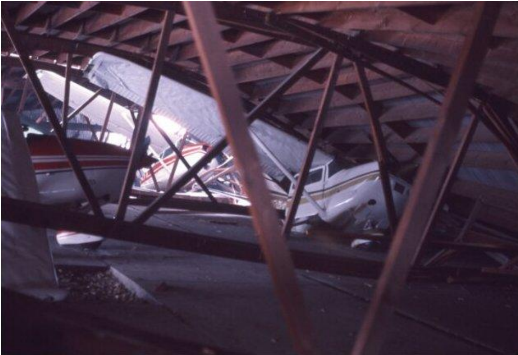
Picture #4B Hangar Collapse
